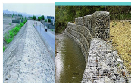
Figure 3b: Flood Protection Bunds and Gabions (www.pixshark.com)
