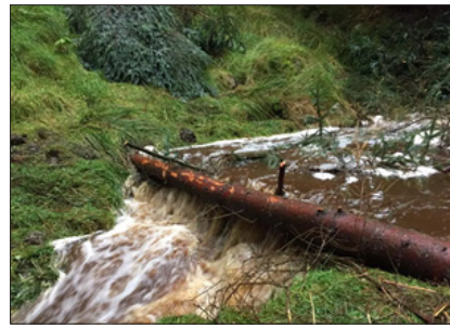
Leaky dam on the River Wharfe during high flow conditions (Yorkshire Dales River Trust, 2018)
