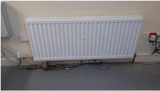
Figure 3 Column radiator located in the kitchen.
