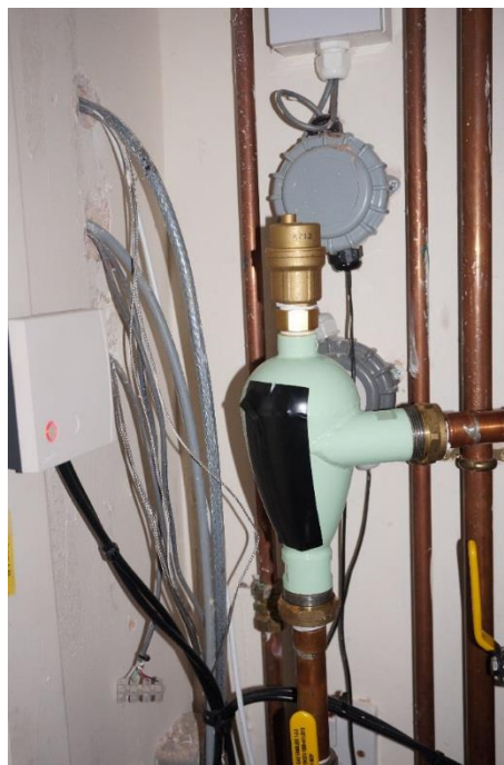
Figure 6 Oxypod® device installed in situ on the primary flow to the boiler.
