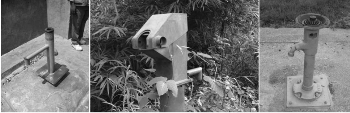
Fig. 1 Broken water infrastructure in Sub-Saharan Africa
