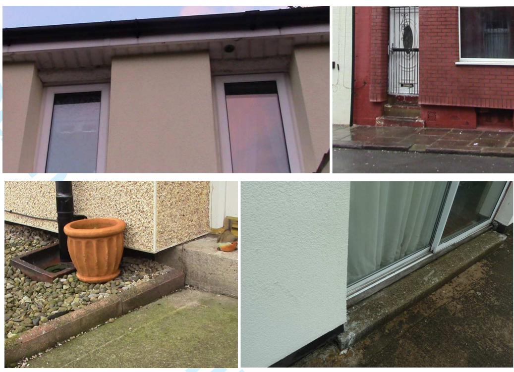
Figure 12 Common EWI details causing thermal bridging
