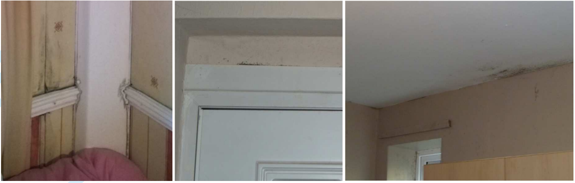
Figure 2 Examples of moisture issues observed prior to retrofit
