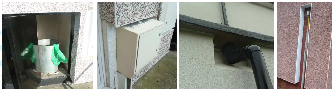
Figure 15 EWI discontinuities at internal bin store and wall mounted gas meter and pipework
