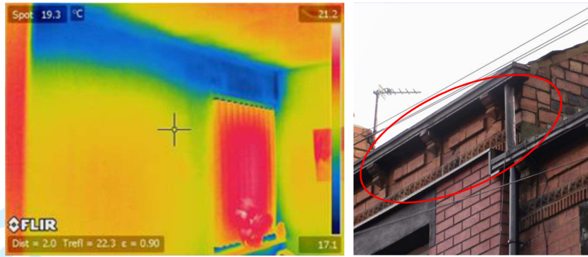
Figure 14 EWI commonly missing at eaves
