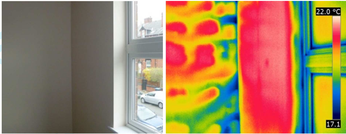
Figure 10 Thermal bypass showing external air entering the dwelling behind the IWI on the external wall under dwelling depressurisation and moving into the void behind the plasterboard on the adjacent internal partition wall.
