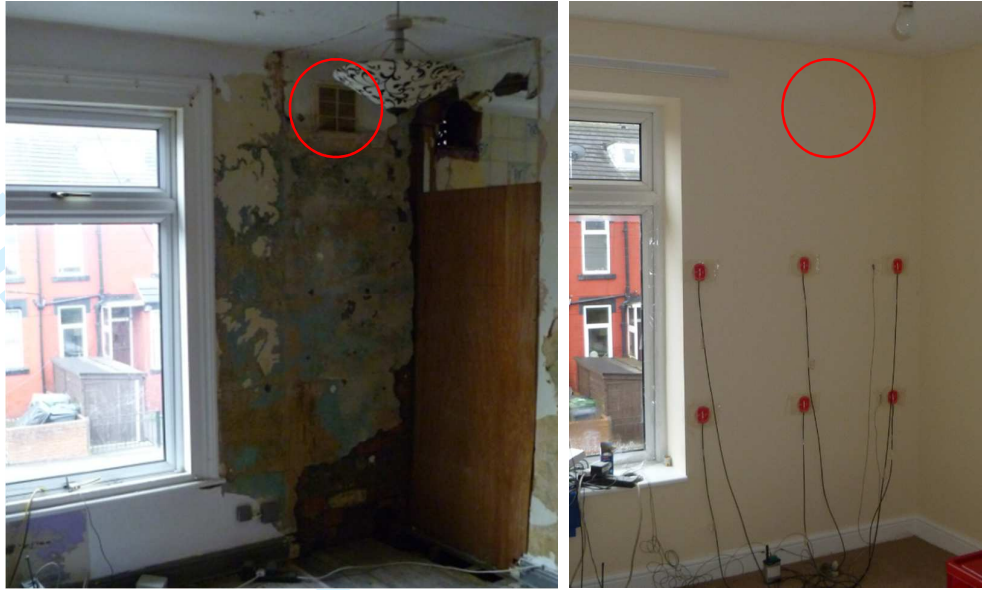
Figure 5 Air brick covered over after IWI installed
