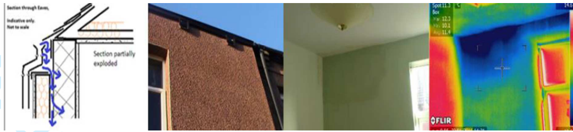
Figure 3 Photographic and thermographic observation of damp and schematic to show route of water ingress behind EWI
