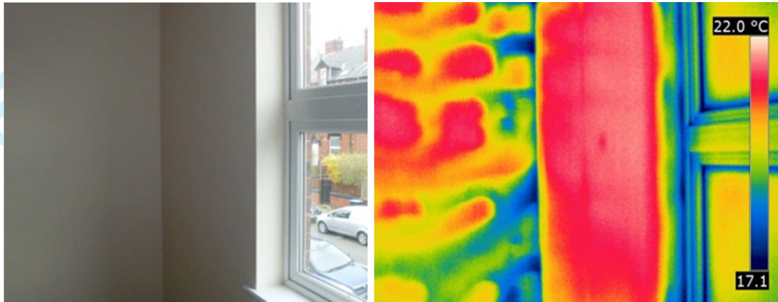
Figure 10 Thermal bypass showing external air entering the dwelling behind the IWI on the external wall under dwelling depressurisation and moving into the void behind the plasterboard on the adjacent internal partition wall.
