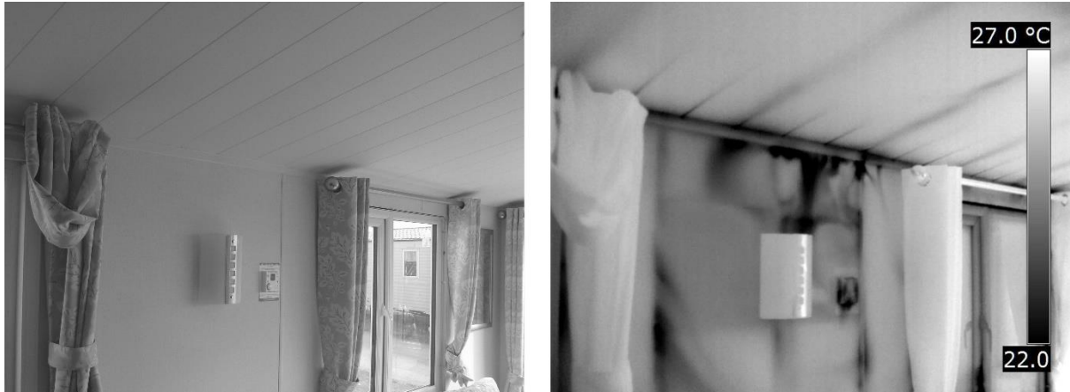
Figure 8 Indirect air leakage around electrical cable runs.
