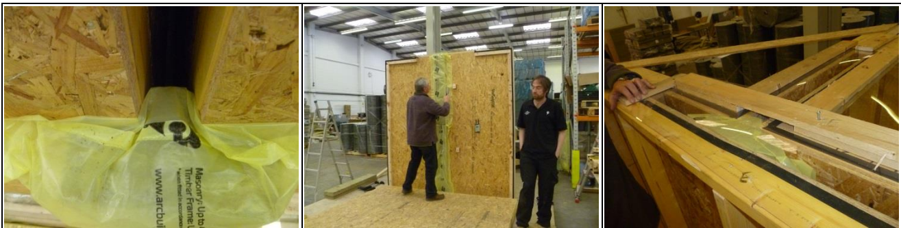
Figure 18 Test 1.4, ARC T-Barrier, 50 mm party wall, 50 mm external wall
