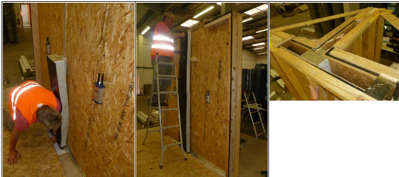
Figure 26 Test 3.7, ARC T-Barrier, 75 mm party wall, 100 mm external wall
