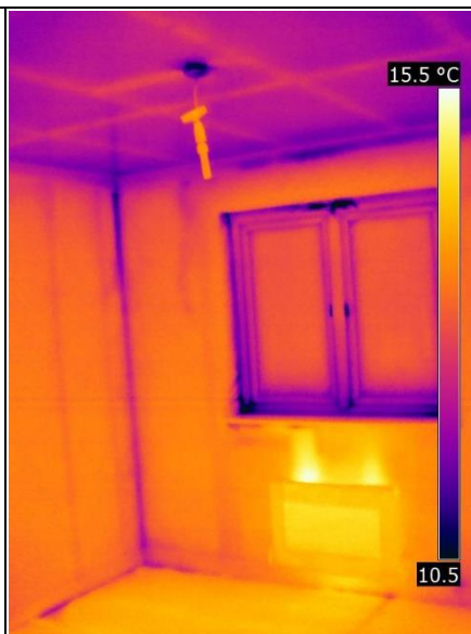
As Bedroom 1; again some air was observed being drawn into the wall panels, but was difficult to detect entering the actual room as it was emerging at the intermediate floor perimeter at room temperature (so not showing up on the thermal camera).
