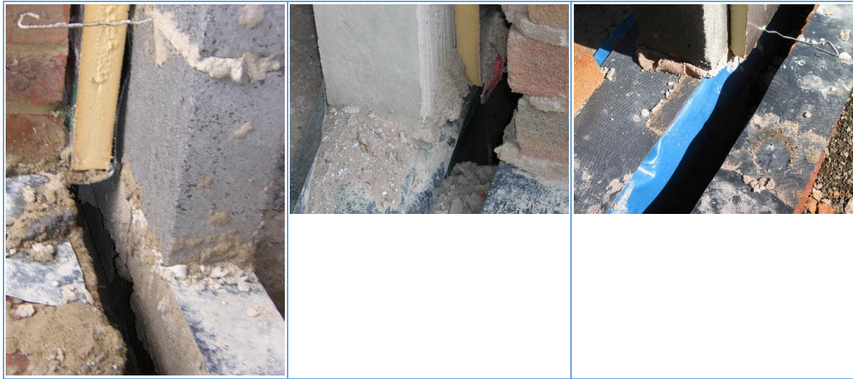
Figure 26 Partial-fill insulation not extending below ground floor level
