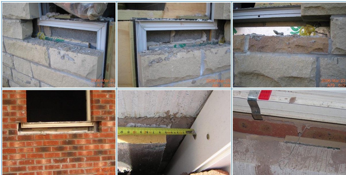
Figure 24 Gaps around partial-fill insulation boards at openings
