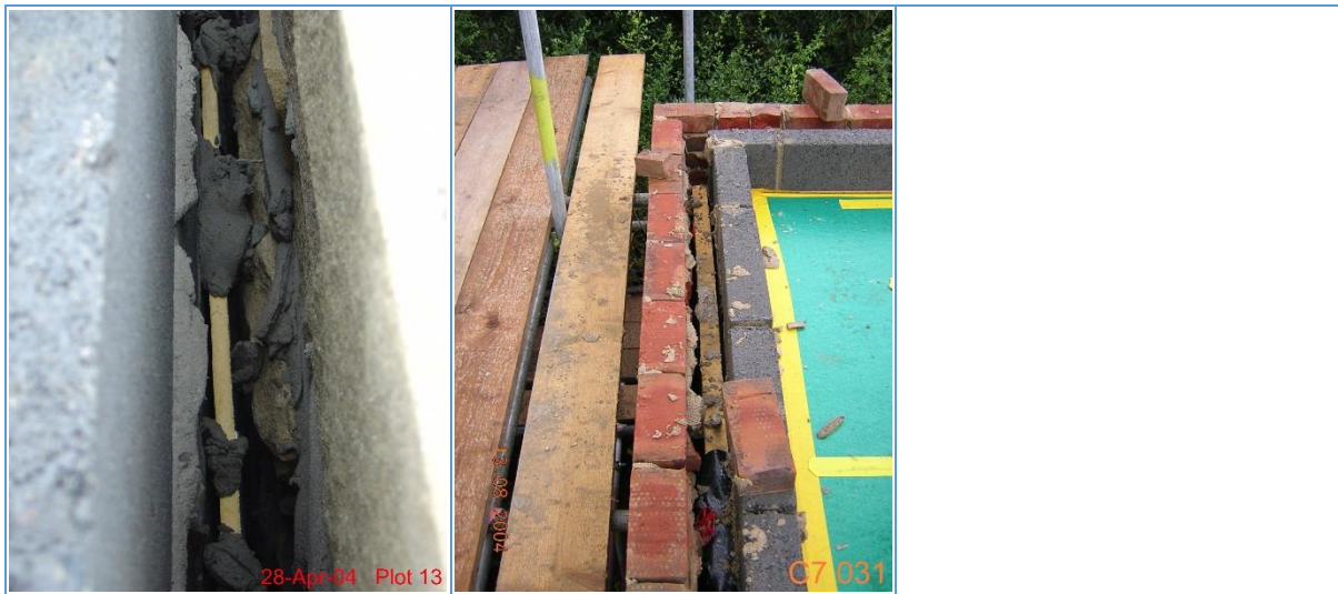
Figure 22 Partial-fill insulation affected by mortar snots
