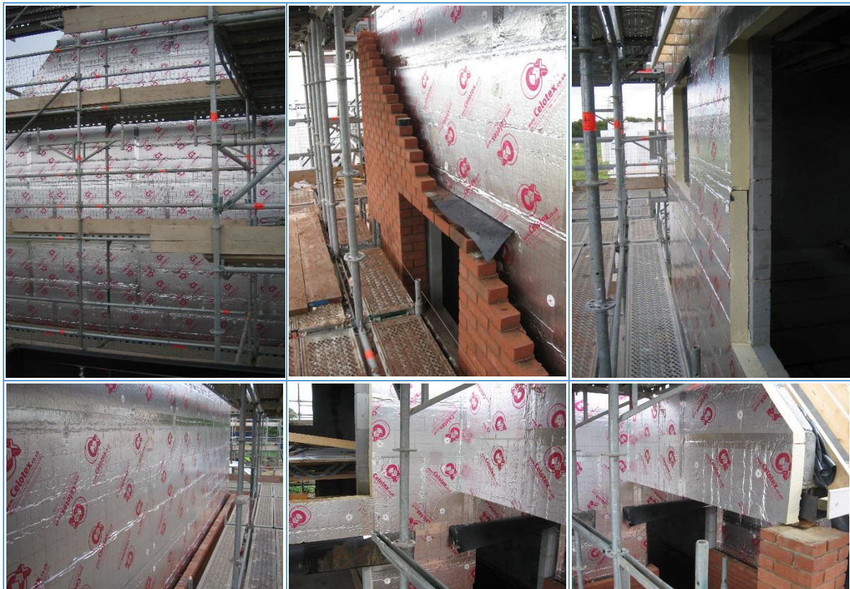
Figure 19 Partial-fill insulation being installed in a thin-joint masonry construction prototype house in York.
