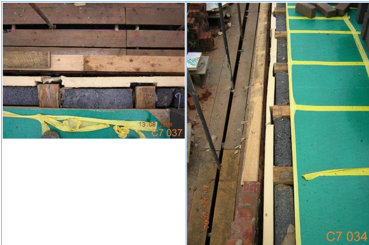
Figure 28 Missing/displaced insulation due to wall protrusions
