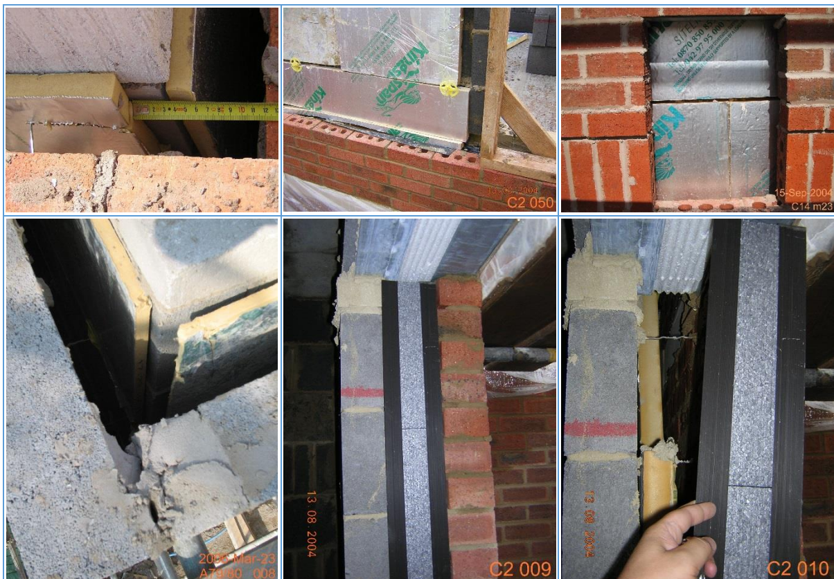
Figure 23 Gaps between and around partial-fill insulation boards
