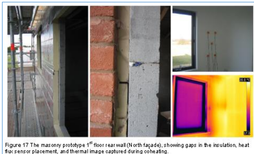
Figure 20 Measured discrepancy in performance due to small issues with partial-fill rigid board insulation (Miles-Shenton et al, 2010)
