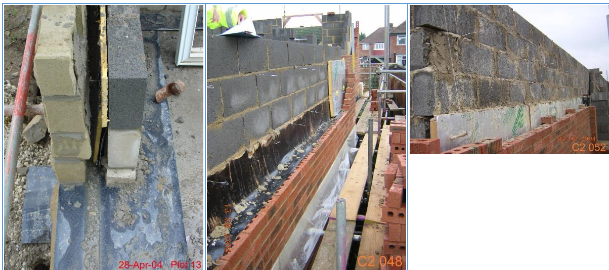
Figure 25 Issues with partial-fill insulation around cavity trays
