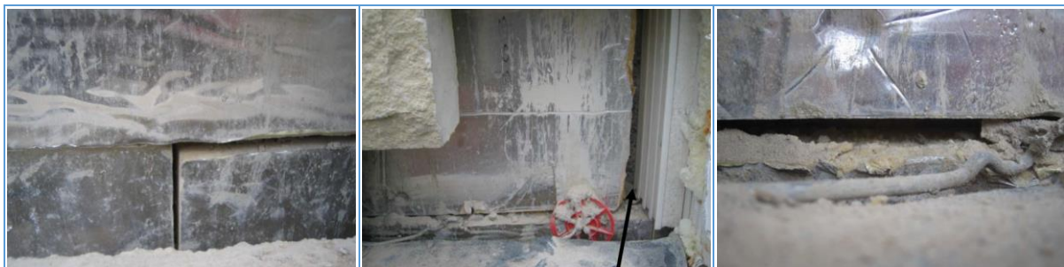
Figure 15 Deconstruction allowing gaps to be seen in the partial-fill insulation, from Wingfield et al., 2009.
