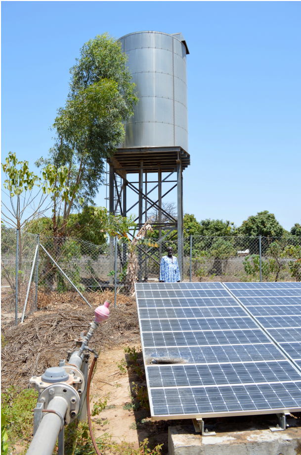
Fig. 4 Kartong central water supply Dudu Sanyang in front of the central water supply's tank and solar system (Source: Author's own photography).
