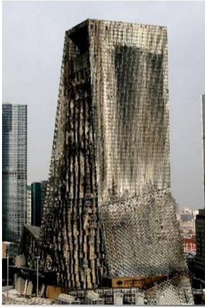
(a) The facade of the fire-exposed building
