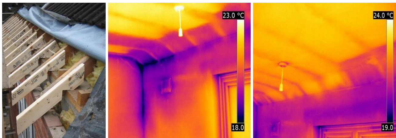
Figure 2-1 Extension of eaves to ensure continuation between the LI and CWI (left) causing thermal bridging on the ceiling eaves (centre) which can be avoided by joining the LI to the CWI (right) [50]
