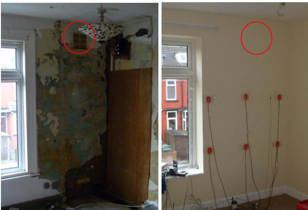
Figure 2-12 Room ventilation (left) which has been covered over by IWI retrofit (right) [110]
