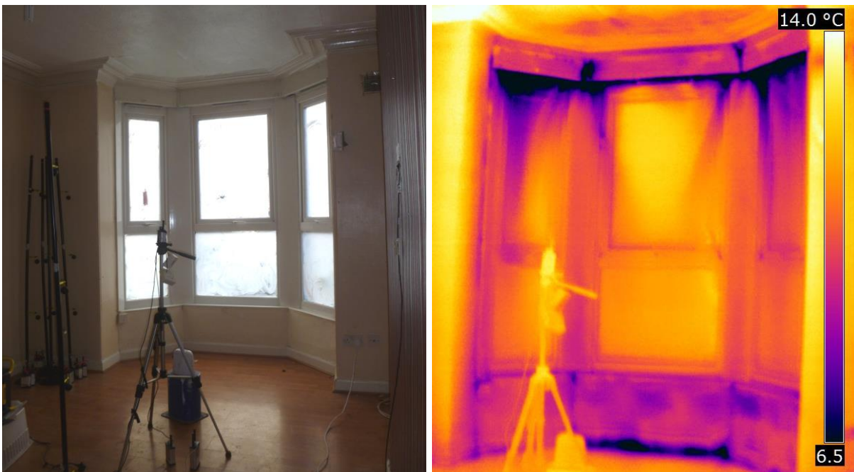
Figure 2-5 Excessive infiltration around window frames after sash windows replaced by casement windows and the resulting gaps have been boxed in, allowing air exchanges via the unsealed tops of the boxing in (unpublished image from [27])
