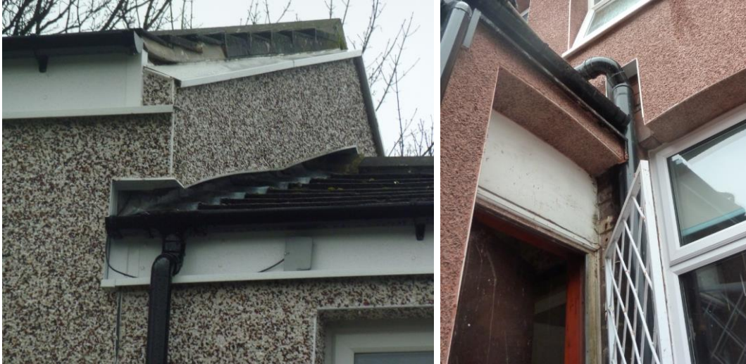
Figure 2-11 Complex construction features causing EWI detailing to create discontinuities in insulation and introduce thermal bridging [110]
