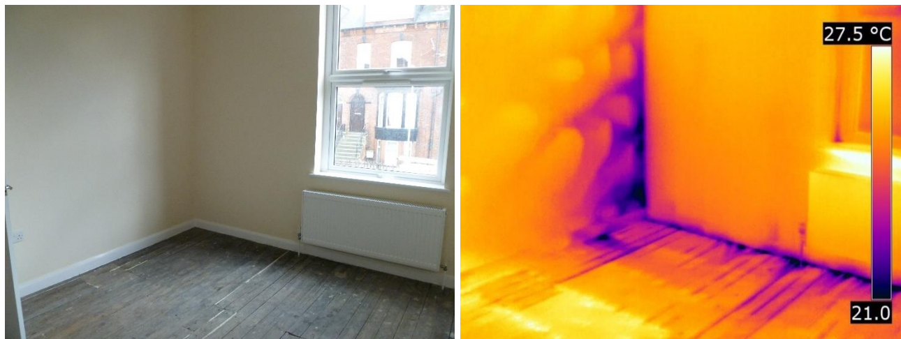
Figure 2-10 Thermal image taken under depressurisation illustrating a direct air leakage around the edges of internal wall insulation which is not adequately sealed [56]
