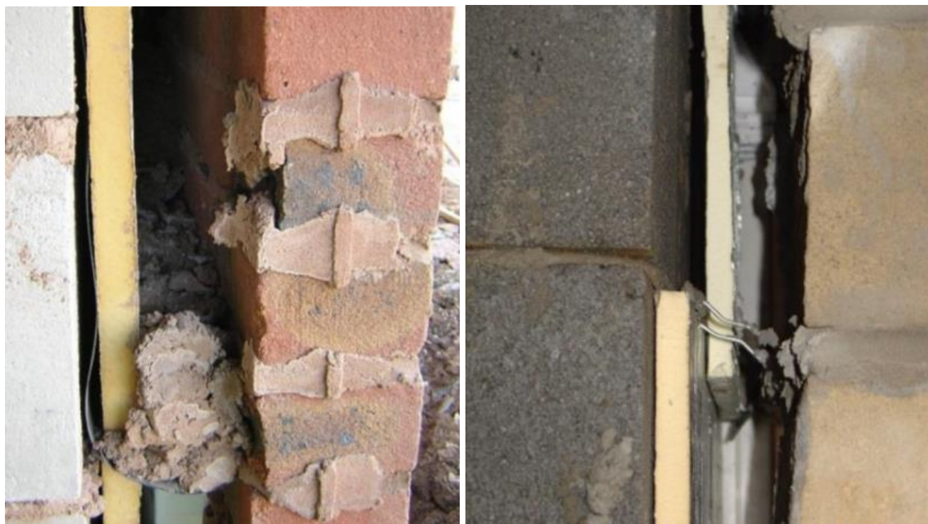
Figure 2-8 Examples of partial fill insulation which is poorly fitted to the cavity inner leaf [44]
