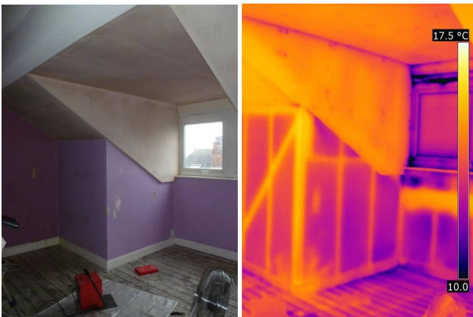
Figure 2-4 Complexity of room in roof geometry and uncertainty around requirements causing partial retrofits and inconsistent fabric performance [27]
