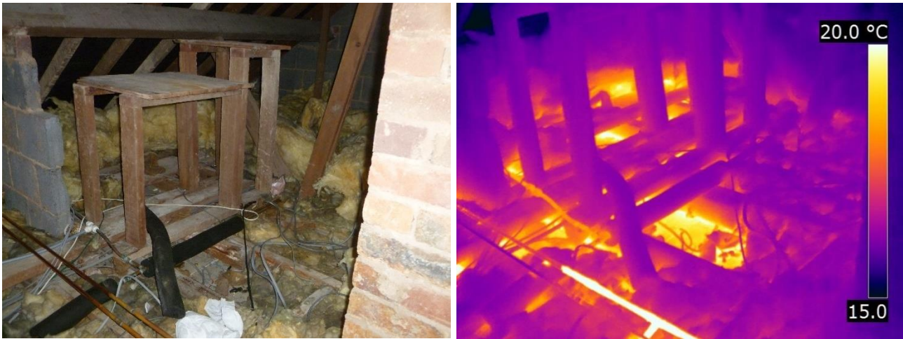
Figure 2-2 Loft insulation removed and piled to one side following rewiring of electrical cables and removal of a water cylinder from the loft space and variability in LI performance
