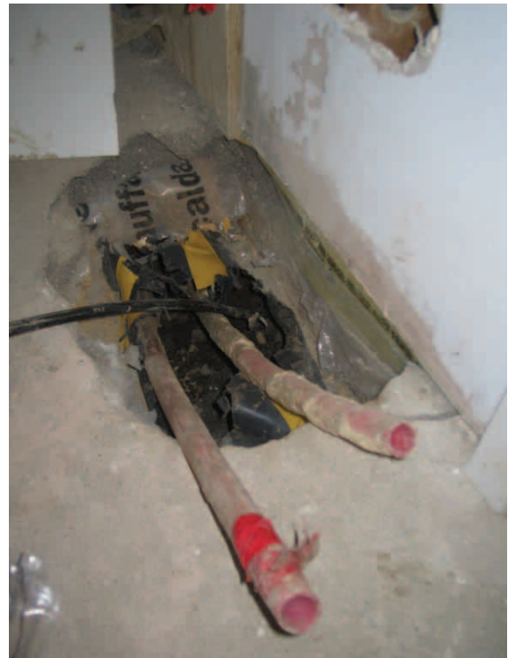
Insulation layer stripped away to enable pipes to be drawn through the floor
