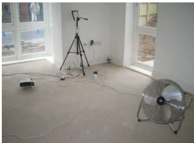
Main test equipment – showing heater, circulation fan and temperature control
