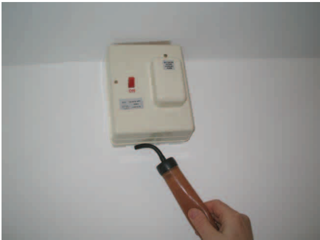
Electricity entry point
