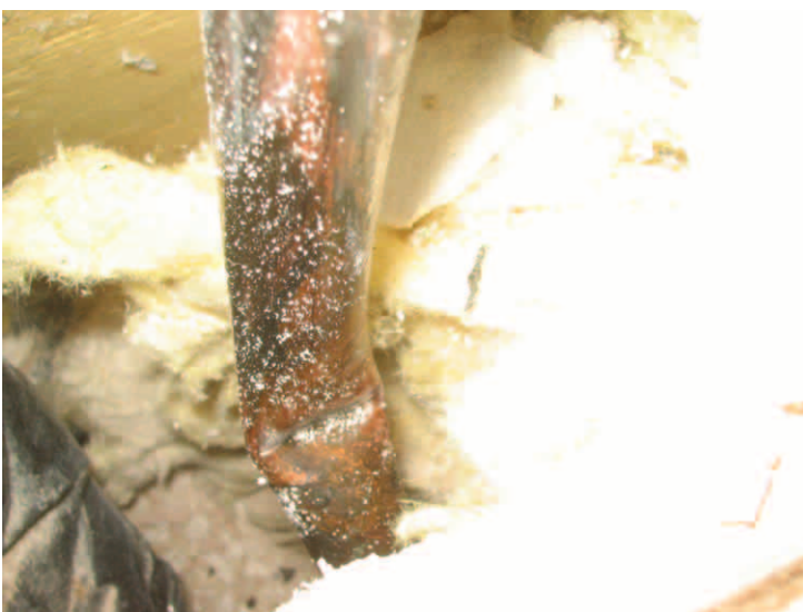
Kinked solar pipe work at wall/floor junction
