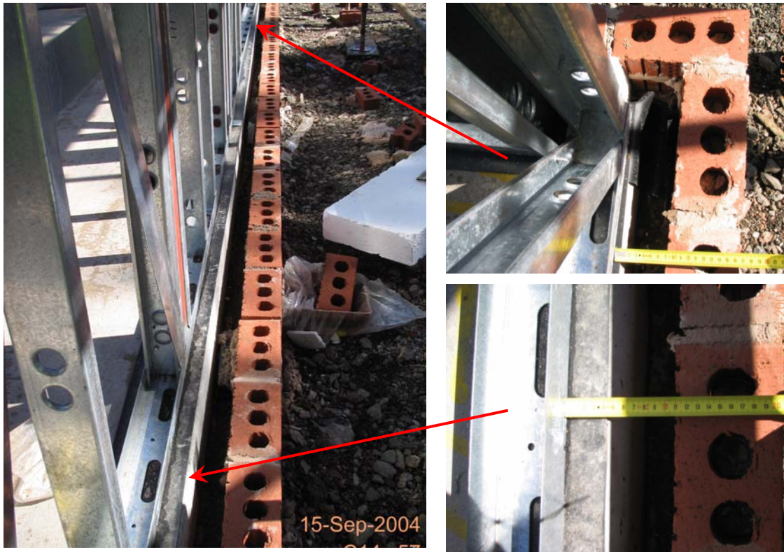
Figure 3.18 Slab not square in steel frame construction.
