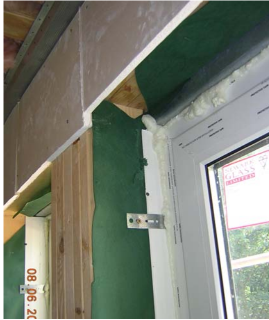
Figure 3.89 Air/vapour control layer not applied to studs – no evidence of layer across lintels and wrapping into head of opening.
