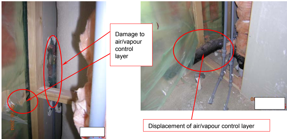
Figure 3.81 Damage to and displacement of the air/vapour control layer.
