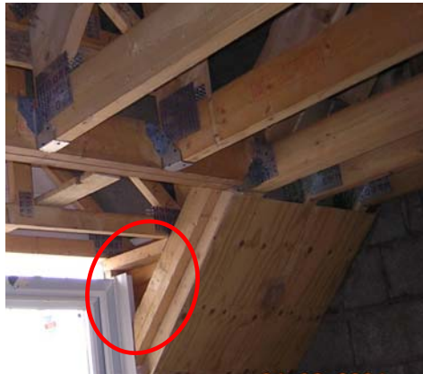
Figure 3.64 Small triangle of external wall difficult to fill with insulation.
