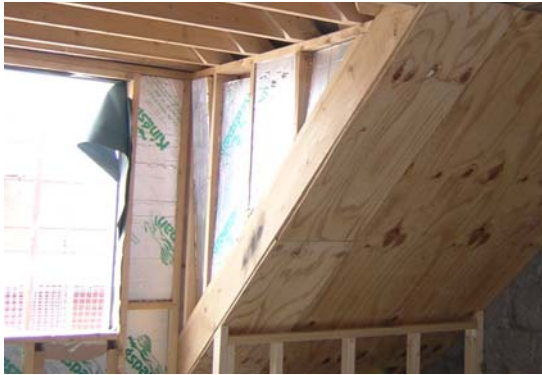
Figure 3.65 Irregular fitting of 35mm insulation boards.
