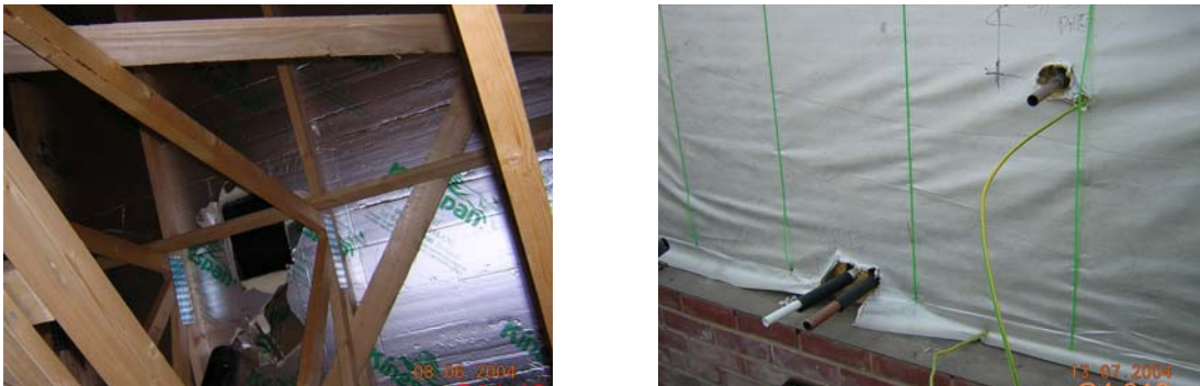
Figure 3.93 Service penetrations through the insulation and air/vapour layers in roofs and walls.
