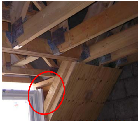
Figure 3.64 Small triangle of external wall difficult to fill with insulation.
