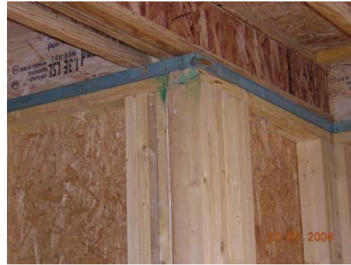
Figure 3.76 High timber concentration at corner post.
