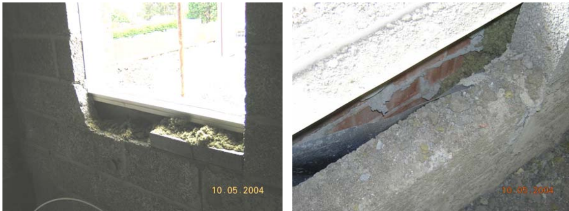
Figures 3.40 and 3.41 Blown fibre, full-fill cavity wall insulation at incomplete sills
