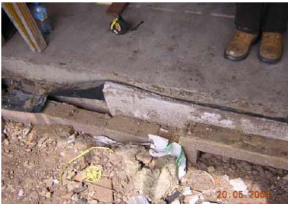
Figure 3.10 Gap in slab edge insulation in timber frame construction.
