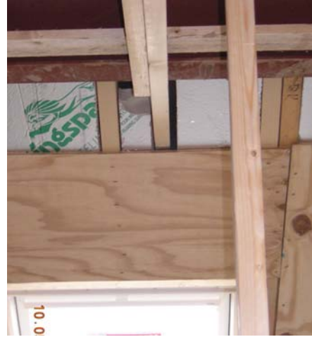
Figure 3.52 Gaps around insulation boards between rafters.
