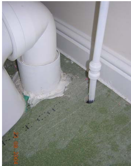
Figure 3.97 Sealing around soil pipe – water pipe yet to be sealed?
