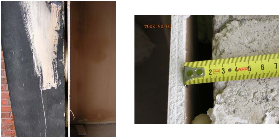
Figure 3.91 Lack of continuity of plaster adhesive to plasterboard lining.
