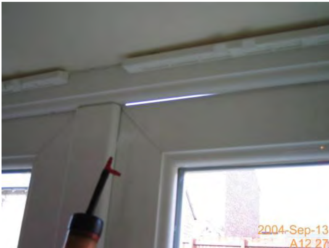
Figure 26 Poorly fitting patio door with visible gap.
