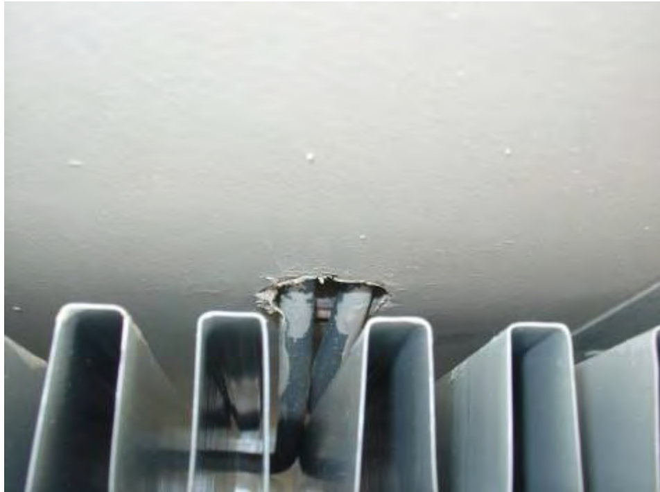
Figure 17 Leaks as pipework penetrates dry-lining behind radiators.
