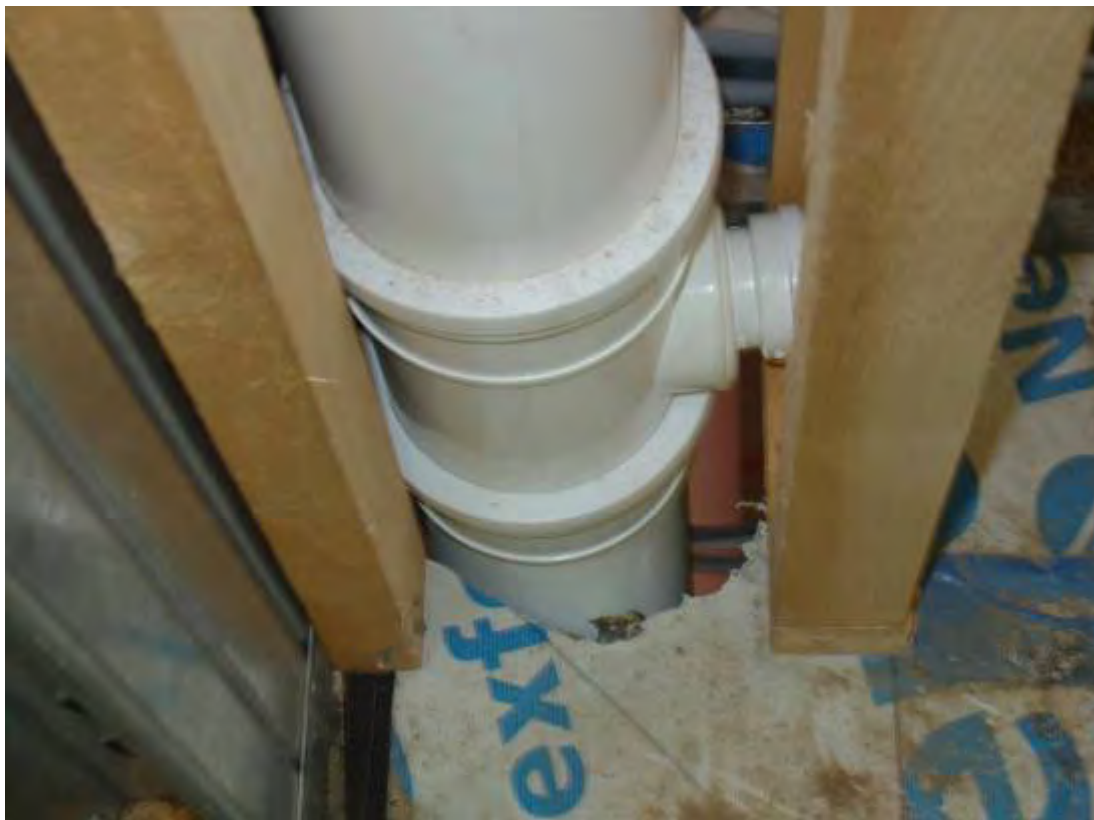
Figure 14 Unsealed soil stack penetrating through intermediate floor.
