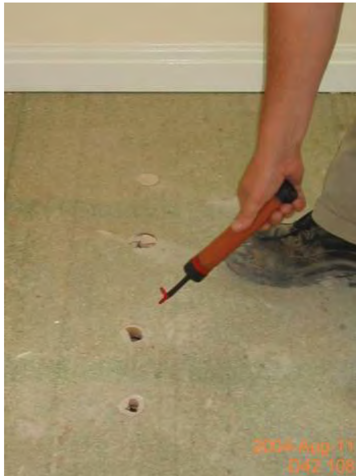
Figure 20 Holes in the flooring panels.
