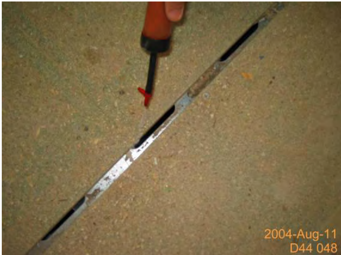
Figure 19 Leaks at the junction between flooring panels.
