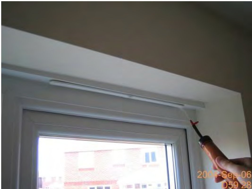
Figure 25 Leakage through poorly fitting trickle vents.
