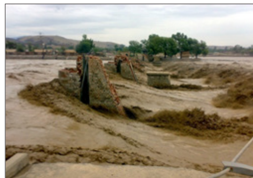
Figure 24: Munda Headworks Structure destroyed after flood 2010 [50]
