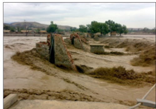
Figure 24: Munda Headworks Structure destroyed after flood 2010 [50]
