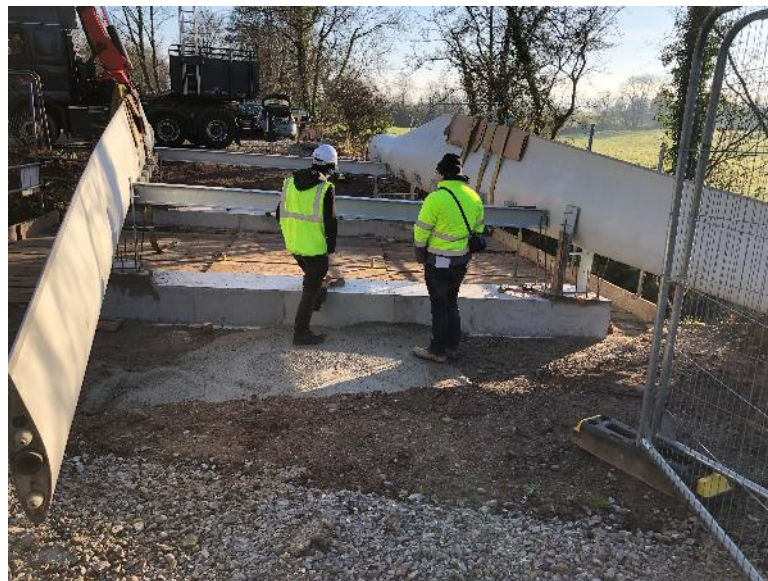
Figure 9. BladeBridge during assembly showing the cradles supporting the blades (prior to installing all the deck beams and plates).
