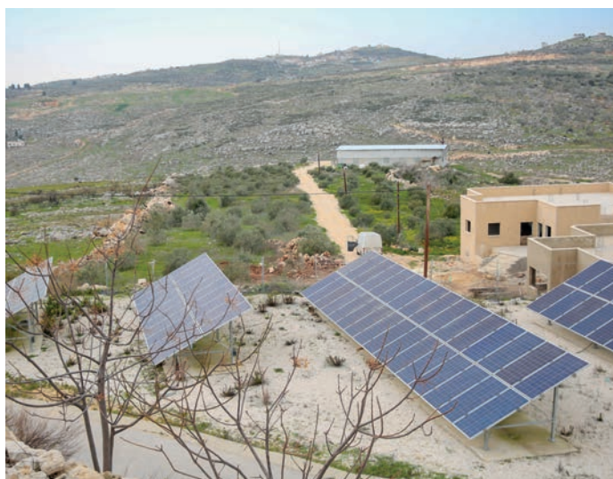
Solar panels on previously unused land now supply clean energy to Ajjah, Palestine. © PENGON
