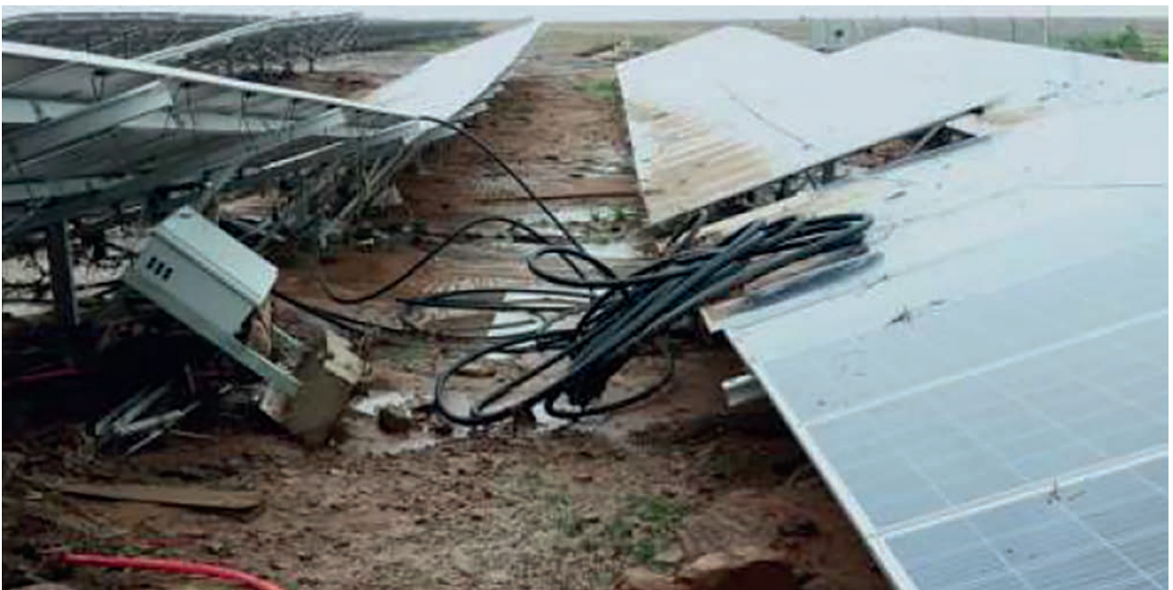
FIGURE 2.3 | DANGEROUS LIVE WIRES POSING A RISK TO PEOPLE AND LIVESTOCK
