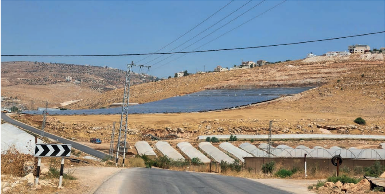
FIGURE 3.2 | GRID CONNECTED SOLAR PROJECT IN TUBAS
